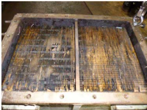
Air Cooler Core before Cleaning
